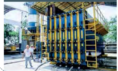
Philippines Battery system
